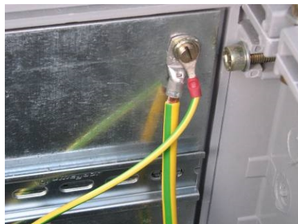
Picture 8 – Grounding point into junction box
